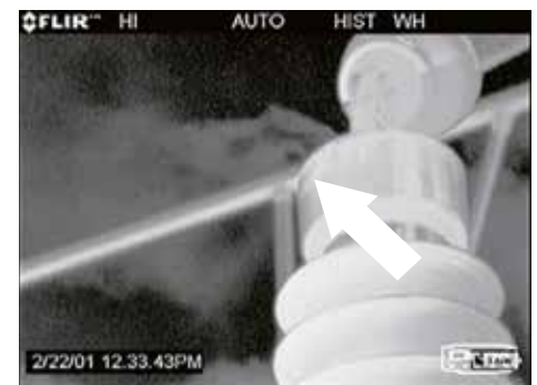
SF 6 leak from a high voltage insulator
